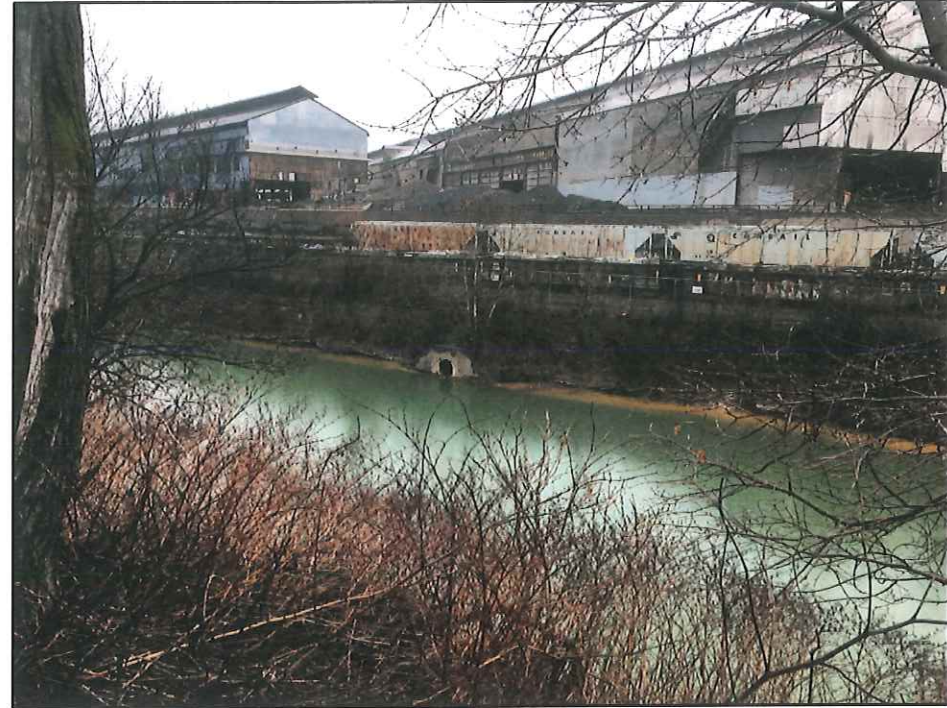
Photograph 1 – View of existing concrete headwall of 48-inch diameter culvert conveying Trib 64495 to Turtle Creek. The enclosed stream culvert is buried nearly 20 feet below existing ground surface. View is facing north.
